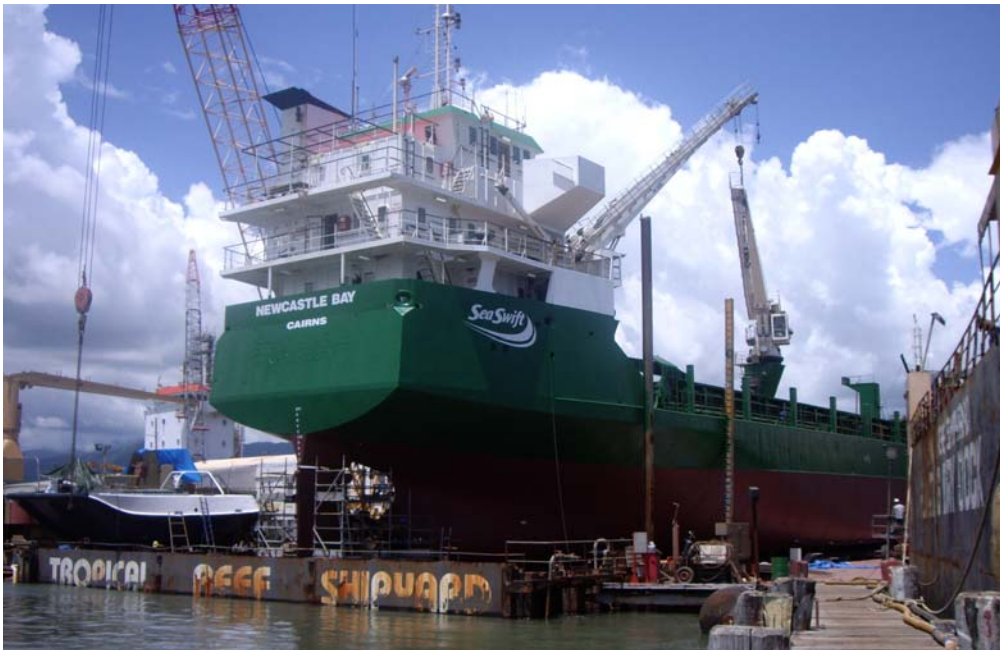
The vessel underwent an extensive refit . The work was conducted by Sea Swift engineering and included work on the main engine, gearbox, stern gear and fwd crane, minor hull repairs and general blasting and painting.
